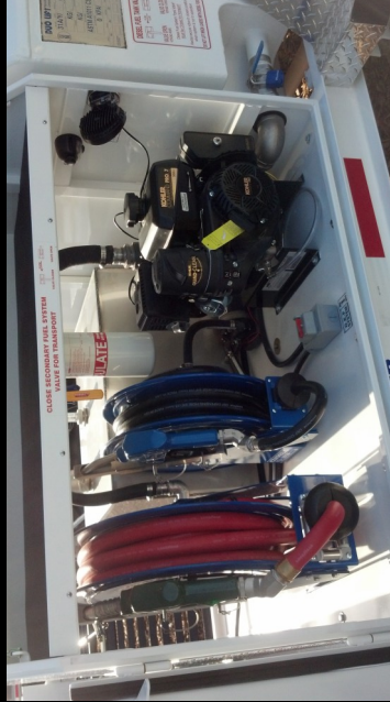
Kohler Powered 30 - 35 GPM Diesel Pumping System with 50 Gallon D.E.F. Tank.
